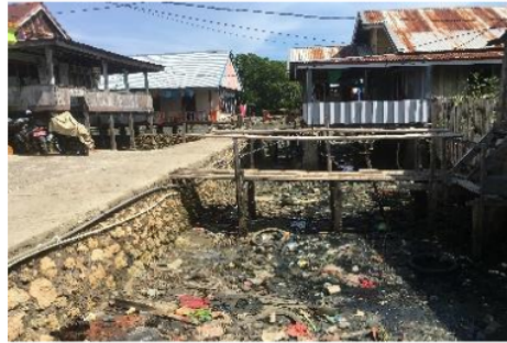
Picture. 14. Condition Drainage in Settlement Patterns group Source: Author, 2021
